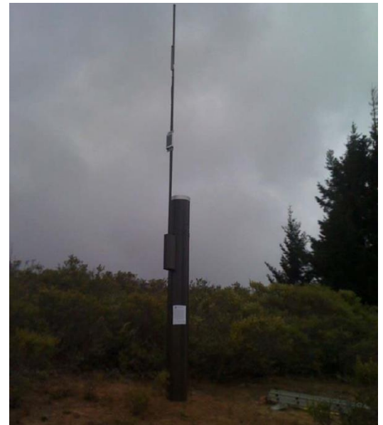
Ventura County project will have ALERT 2 rain gauges similar to the one installed in the San Francisquito Creek watershed as part of a different DWR Emergency Response Grants-funded project (Photo: City of Palo Alto, 2014)
