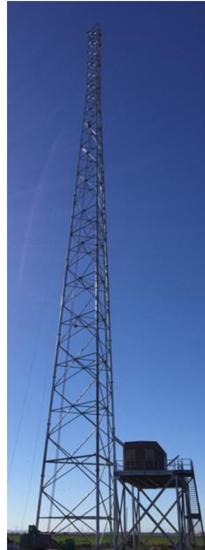
The 300-foot tall Twitchell Island radio communications tower provides interoperable communications for five Delta counties (Photo: DWR, October 2015)
